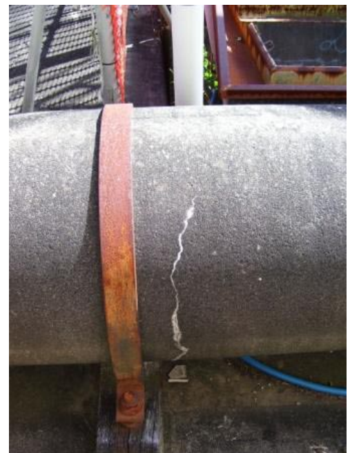
Autogenous healing has filled this 0.5mm wide circumferential crack that has occurred at the bottom of the pipe..
