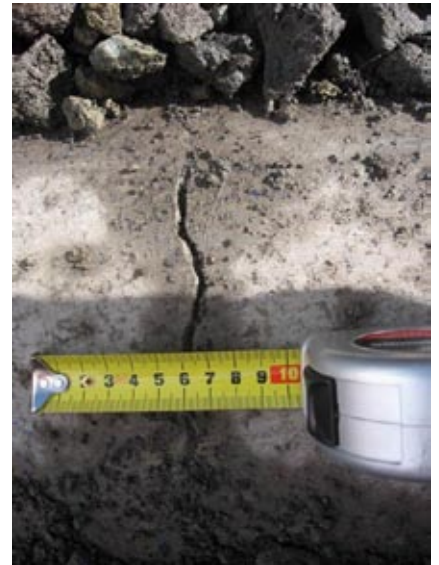
A 6mm crack at the top of a DN300 pipe due to stresses that have resulted from poor bedding
