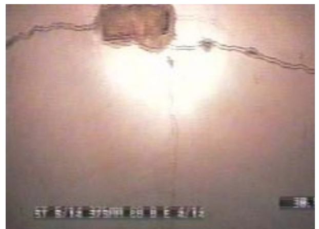
An internal circumferential crack of a DN375 concrete pipe, greater than 0.5mm wide.
