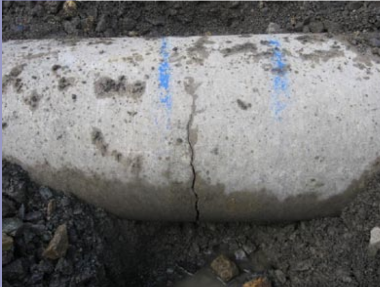
A 6mm crack at the bottom of a DN300 pipe due to stresses resulting from poor bedding.
