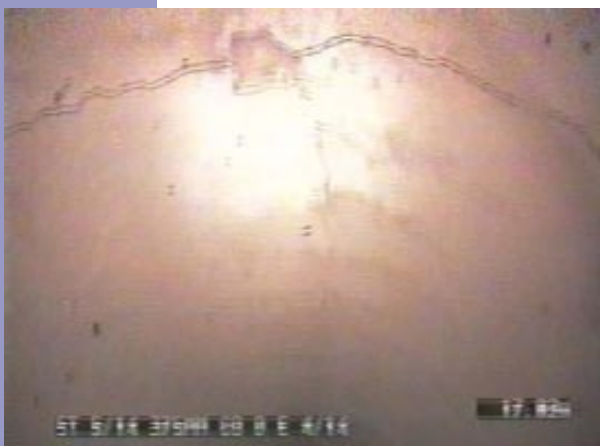
An internal circumferential crack of a DN375 concrete pipe, less than 0.5mm wide.
