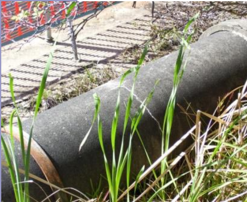
Autogenous healing has filled this 0.5mm wide circumferential crack that has occurred at the top of the pipe.
