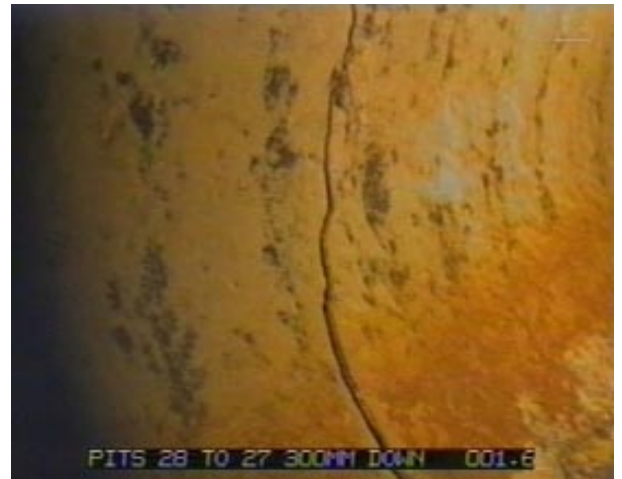
An internal circumferential crack of a DN300 concrete pipe, greater than 0.5mm wide.
