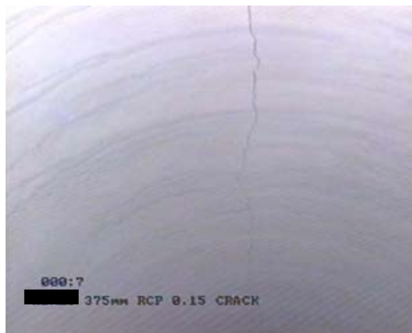
A 0.15mm crack at the obvert of a DN375 pipe tested for proof load. This is acceptable in accordance with AS/NZS4058
