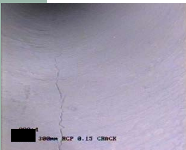
A 0.15mm crack at the invert of a DN300 pipe tested for proof load. This is acceptable in accordance with AS/NZS4058
