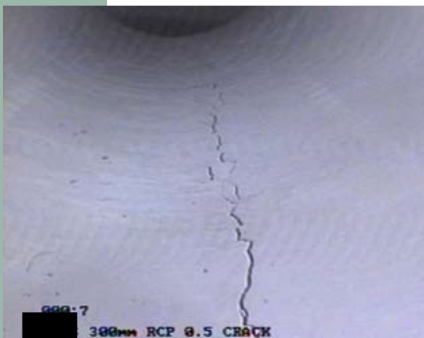
A 0.5mm crack at the invert of a DN300 pipe, possibly caused by overloading of the pipe
