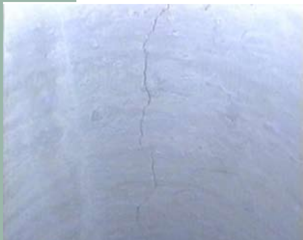
A 0.15mm crack at the obvert of a DN300 pipe tested for proof load. This is acceptable in accordance with AS/NZS4058
