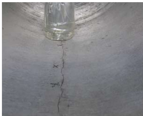
A 0.3mm crack at the invert of a DN450 pipe.
