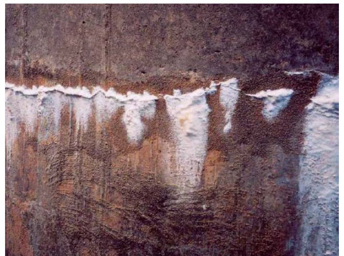
Autogenous healing at an advanced stage on a water retaining concrete structure
