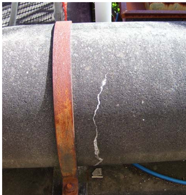
The white line signifies autogenous healing on this exposed concrete pipe
