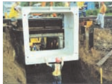
Above: The boxes being "craned" into position. Note the one meter distance from the track to the culvert. Box jacking underway.
