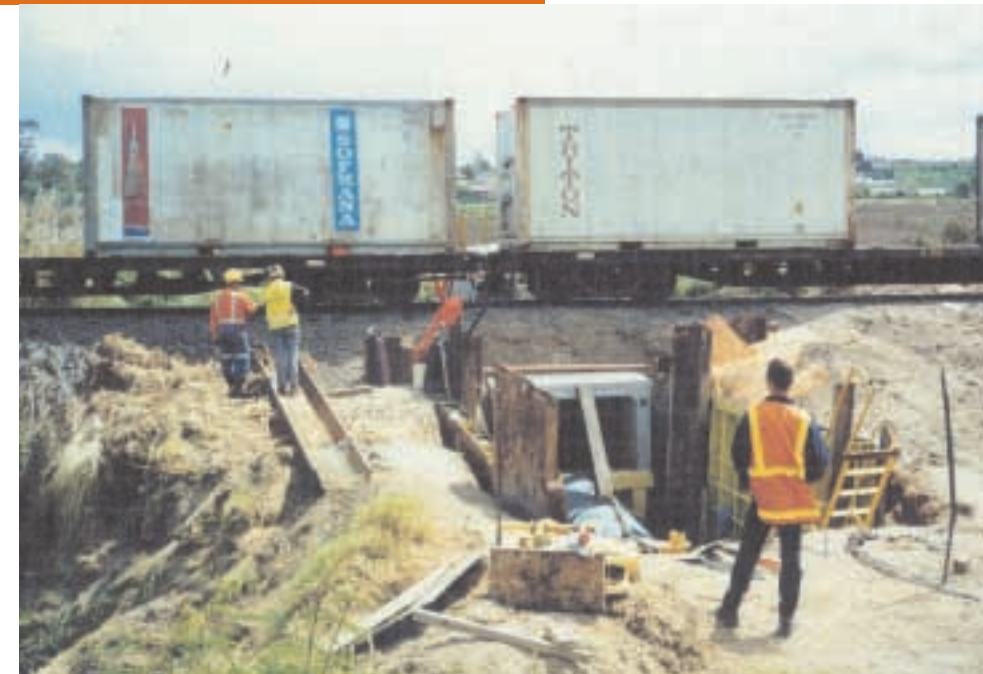
Above: A real success – throughout the project railway use continued. Here a train makes its way from the Port of Tauranga to Auckland.
