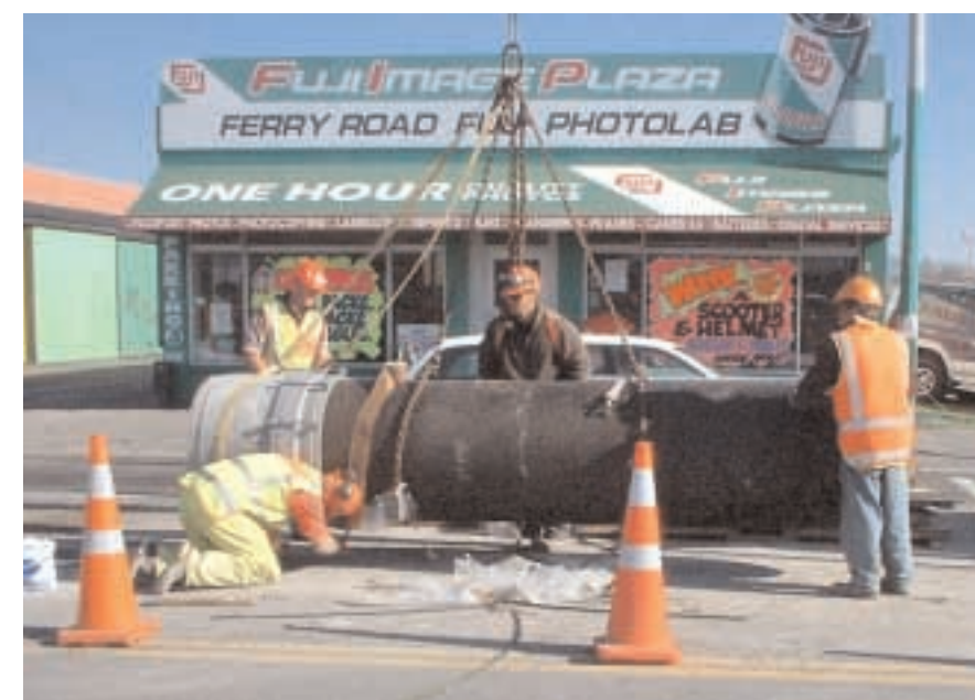
Top right: The 750 diameter valve (2.1m in height) being lifted into the trench.
