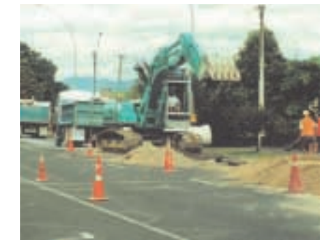
Above: Brown Drainage Limited taking extra care to get the job right.
