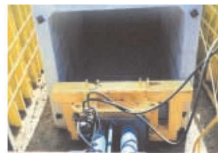
Right: Jacking continues with post-tensioned stressing cables to hold and secure boxes in place.
