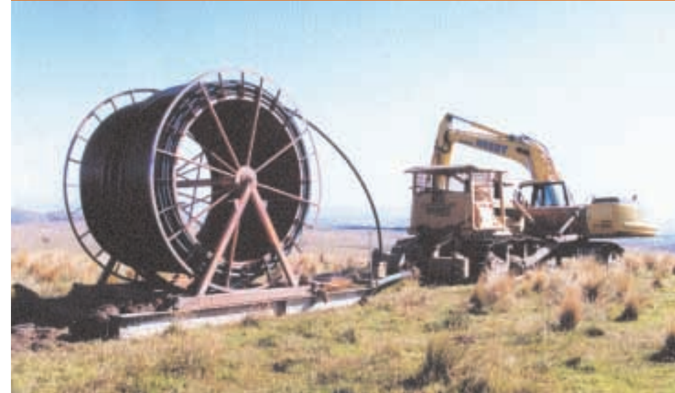
Left: MDPE pipe on a specially constructed Marley coiler being pulled by a D6 bulldozer and assisted by a 20 tonne excavator.
