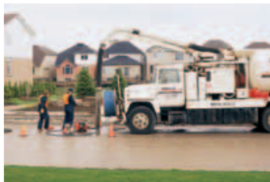
Humegard™ unit being emptied by a vacuum truck
