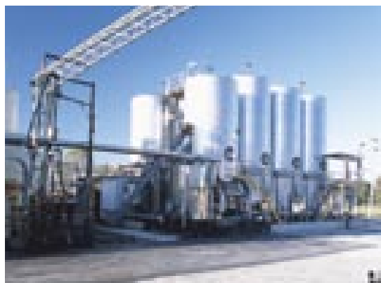
The ability of Humeceptor™ to completely capture spills during both dry weather and wet weather make it an essential risk management tool for industrial facilities.
