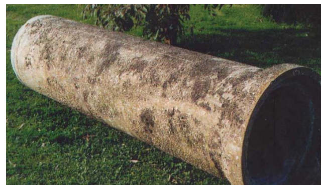
A reinforced concrete pipe retrieved after 50 years service in the Brisbane River - as sound as a new pipe
